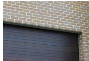
Brick infills above external openings including garage to "face brick" cladded walls.
